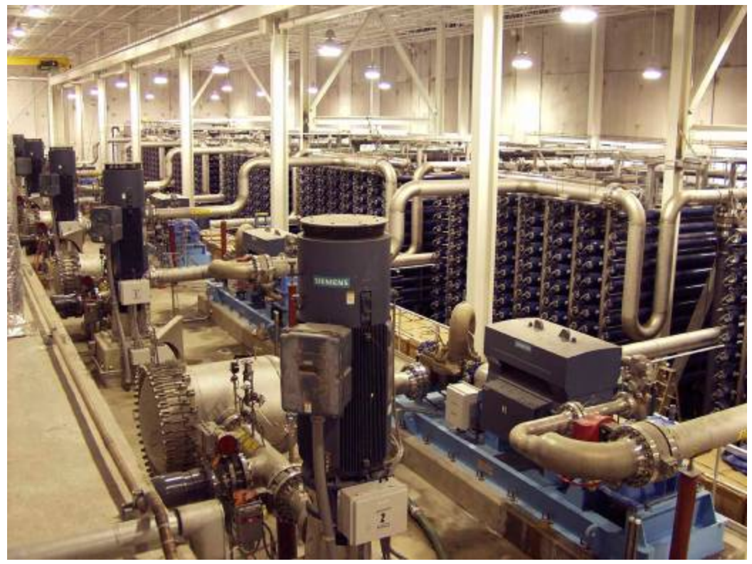
Tampa Bay Water Desalinization Facility
